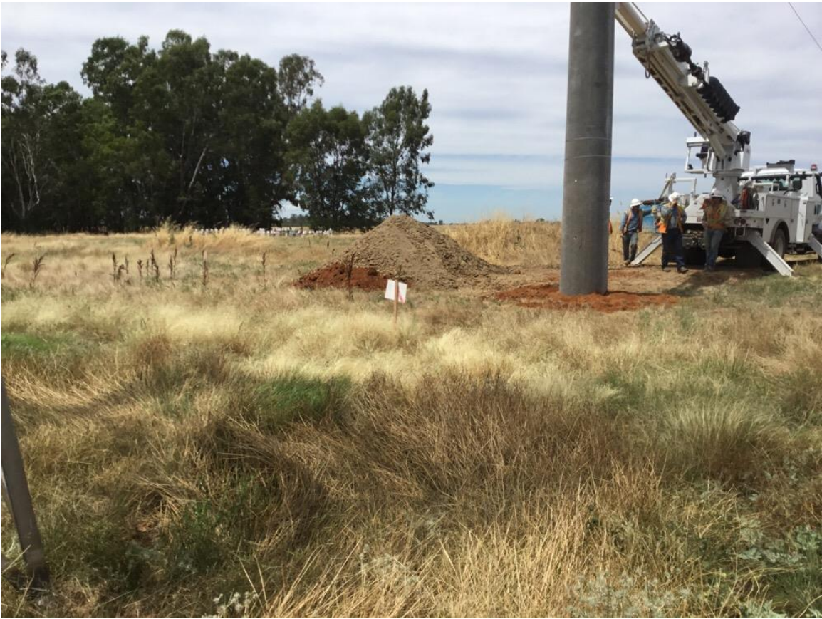
Photo 2: Dirt spoil pile staged outside of clearly marked vernal features in accordance with SWPPP BMPs.
